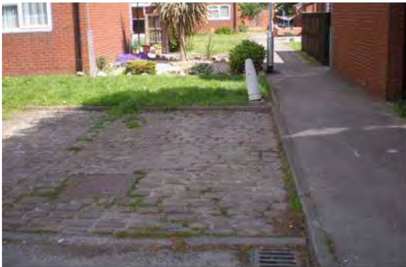
Stone sett paving adds texture to a parking area, but needs to be better maintained to look its best
