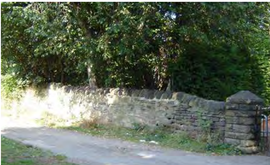
Stone walls are an important feature in the area. They have not always been maintained with the appropriate type of pointing.
