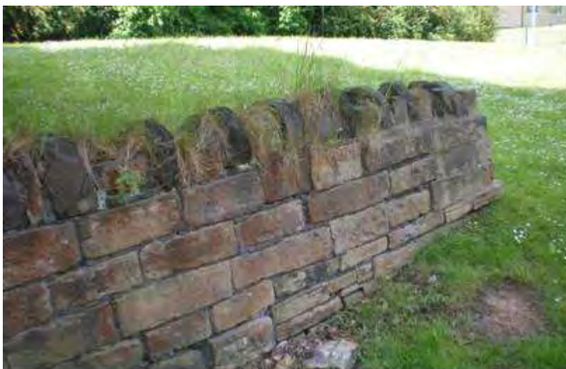
Retaining wall by Lawns Lane adds character to an otherwise ordinary grassed area
